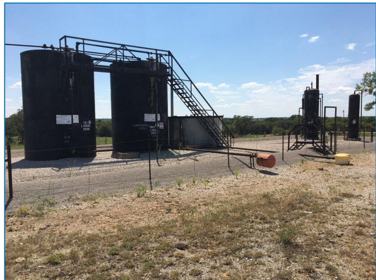
Figure 2. Tank battery and related production equipment, Mitchell 1-12 well, Carter County
